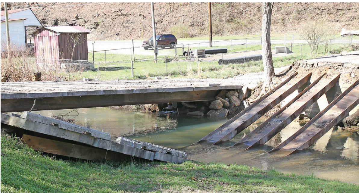
This bridge on Elk Creek collapsed late Friday night/early Saturday morning. County Judge-Executive Tommy Harmon and the road crew had a temporary bridge constructed within hours.
